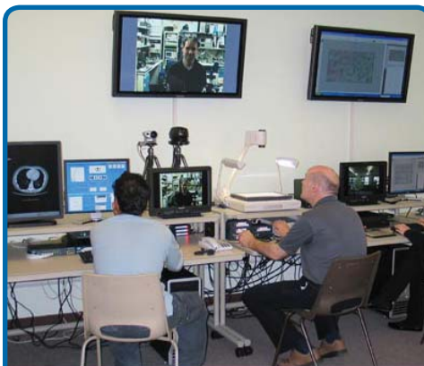
TELESYNERGY® installation in Beaumont Hospital, Dublin.
